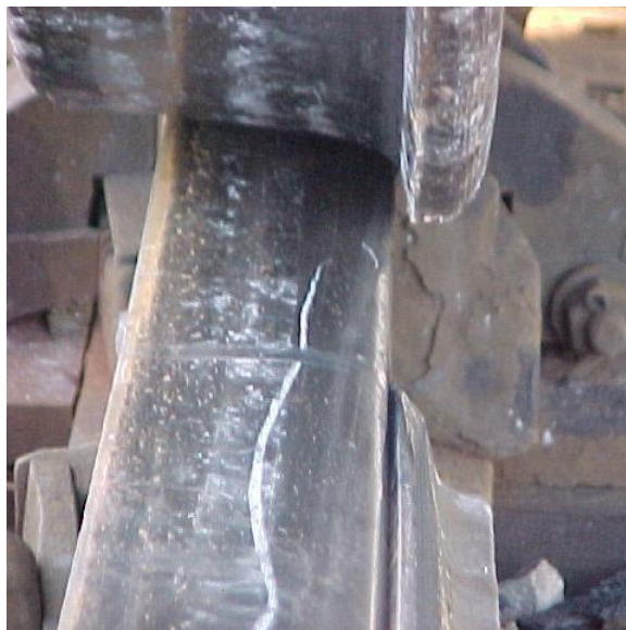
The worn flange is tracking close to the stock rail, approaching a gapped point
